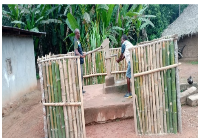
In River Gee, HAC members successfully advocated local leaders to repair and fence a hand pump
